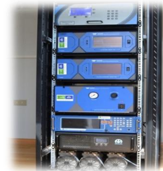
Gas analysers and Gas flow control system
