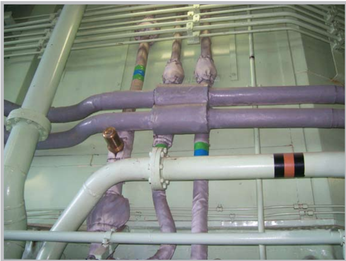
Conductions of boilers shielded by asbestos coating
